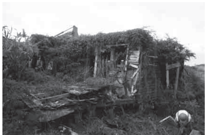
9 (top). The Phase 3 addition prior to rubbish and vegetation removal.
