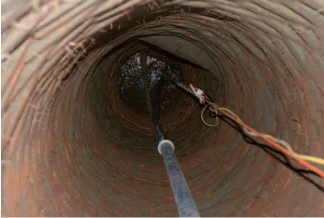
5.7. Looking down into the well at 3 Pipitea Street as it was being drained. Two large beams can be seen in the wall of the well and another beam of wood, possibly just lodged there, lies across the middle.
