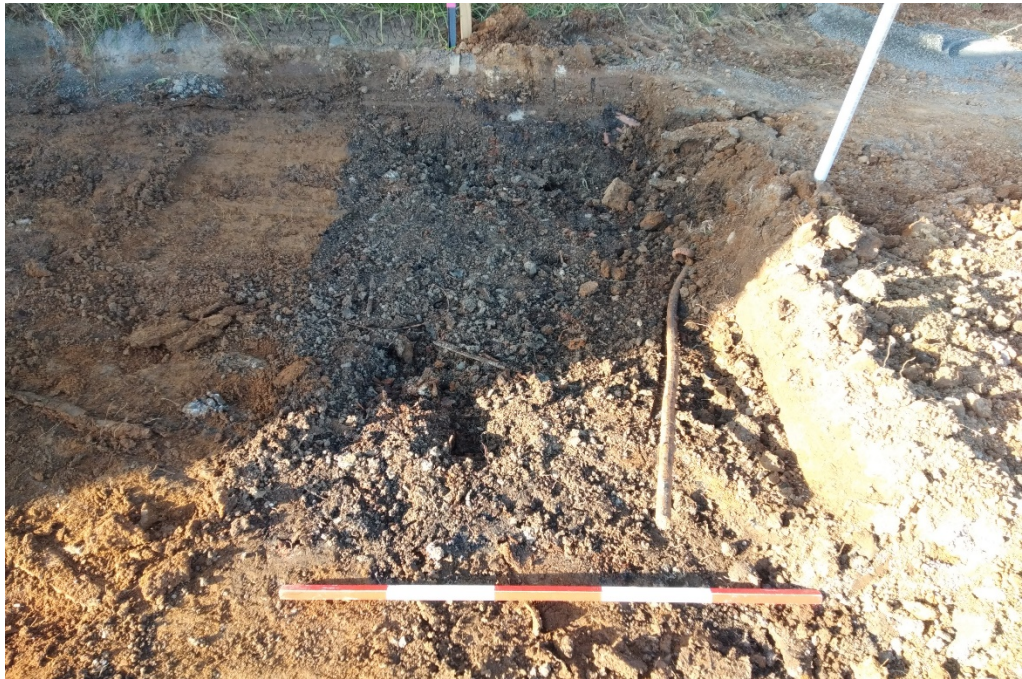
Figure 5. Pit in south of building platform for Units 15-22 containing demolition material from farm buildings
